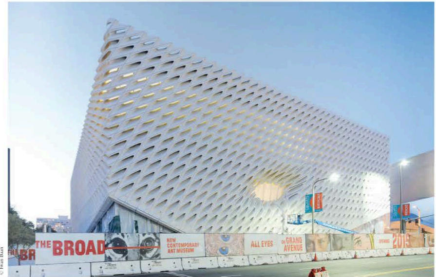
The Broad Museum under construction on Grand Avenue in downtown Los Angeles
